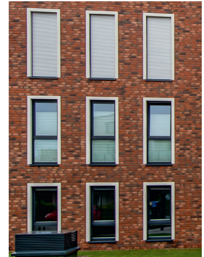
The wild brickwork bond is popular because its timeless look suits many different architectural styles.
