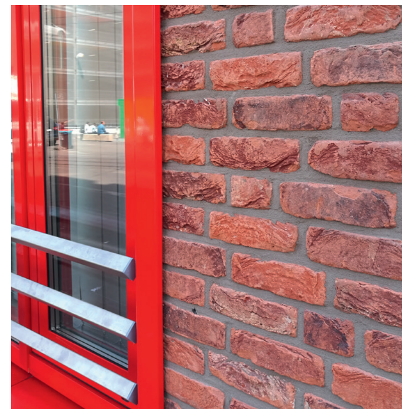
Protruding aluminium window frame
